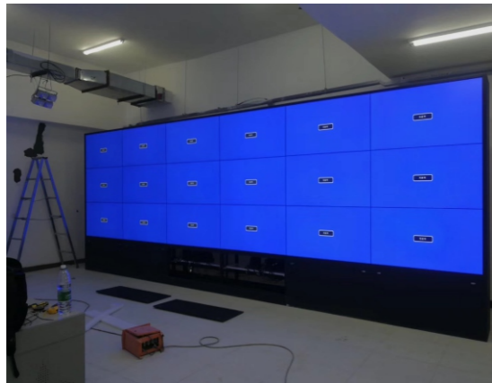
◆ Shanghai shopping mall monitoring room
